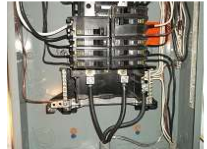
Improperly Wired Subpanel
