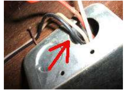
Missing Wire Bushings
